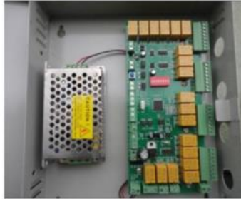
Main Control Box * 1
